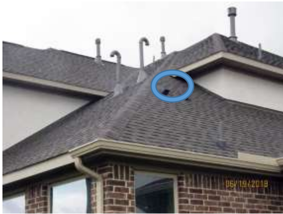
General area of incoming moisture
