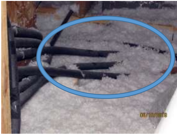
Area in attic affected by leak
